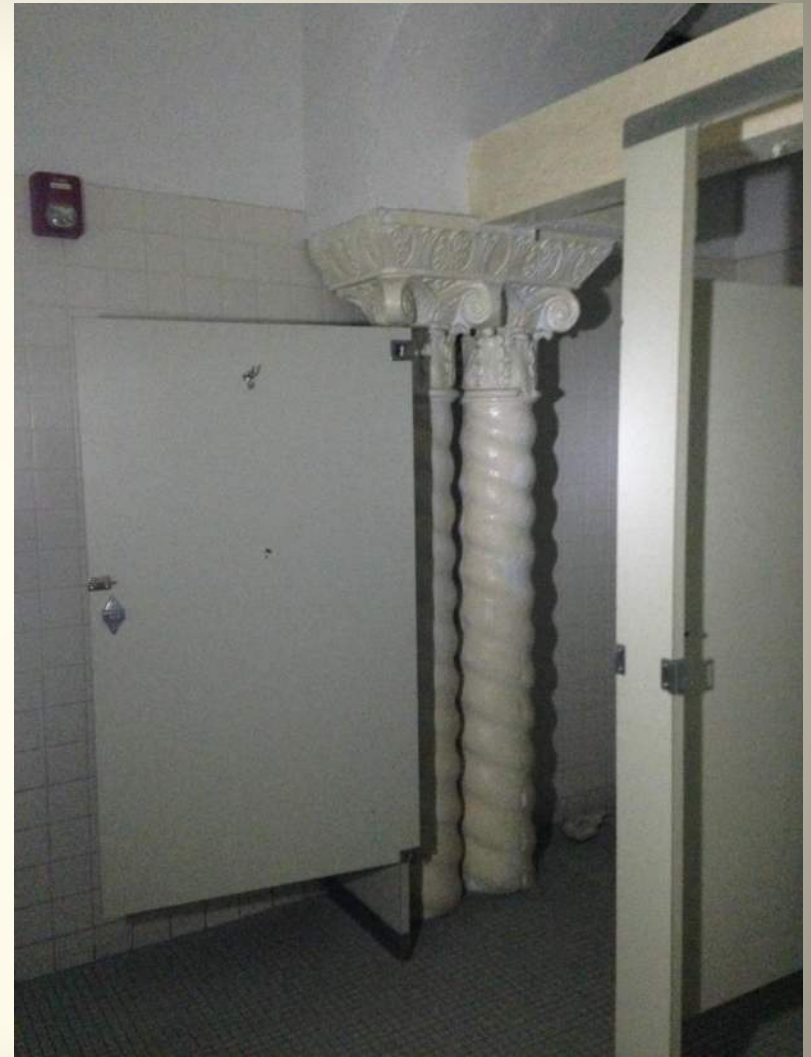
Solomonic Columns now located in the restroom. Due to the change in floor slope, the bases are now below the floor slab.
