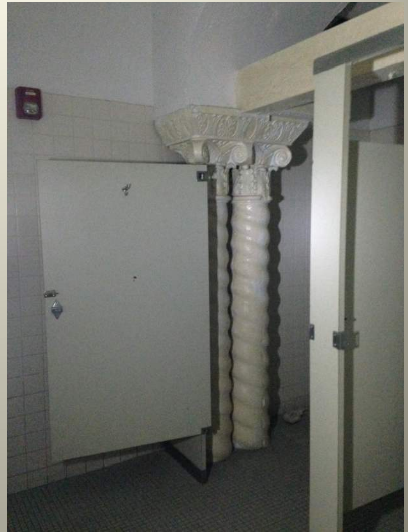
Solomonic Columns now located in the restroom. Due to the change in floor slope, the bases are now below the floor slab.
